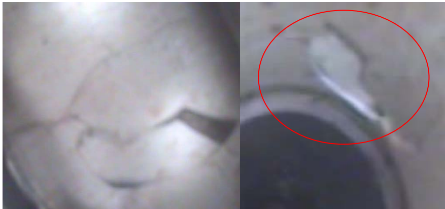
42220019 - Crack in casing at approximately 11.5 m depth.
