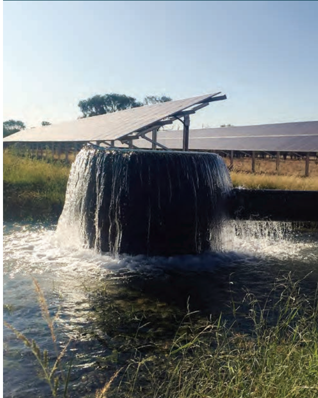
FIGURE 9.3 An industry-first installation of a 55 kw submersible pump driven by combined 100 KW solar and 110 kVA diesel generator at the Gill family's 'Waterloo' Narromine, NSW. © Jon Welsh
