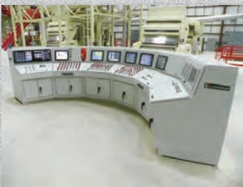
Controls and Control Systems
