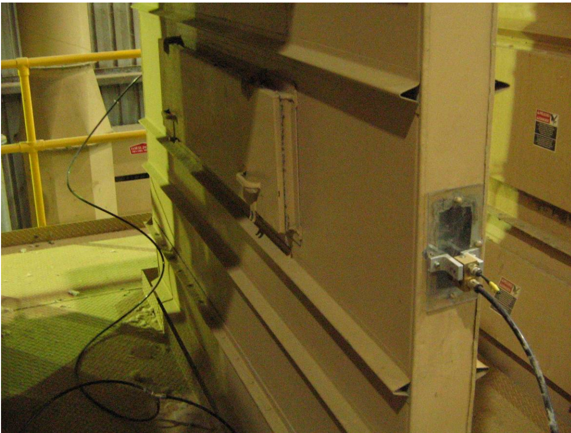
Figure 2 – Nozzles installed into ducting between horizontal pre-cleaning machines at Auscott Warren’s gin
