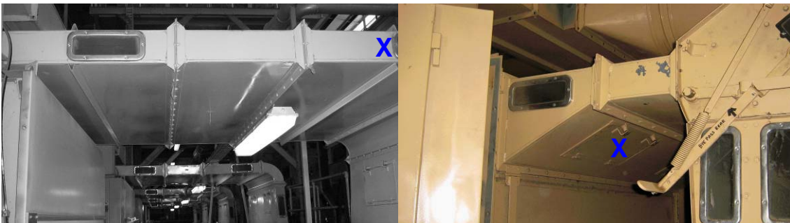
Figure 3 – Nozzles installed into gin ducting at Auscott Warren’s gin between gin and lint cleaner at positions marked with X; (a) 2.0 m from lint cleaner condenser; (b) 500 mm from lint cleaner condenser
