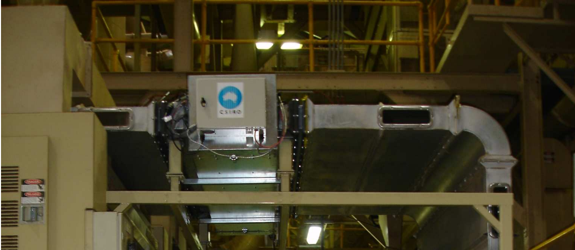
242 FIGURE 9. Position of the device in ducting between the gin stand and first lint cleaner. 243
