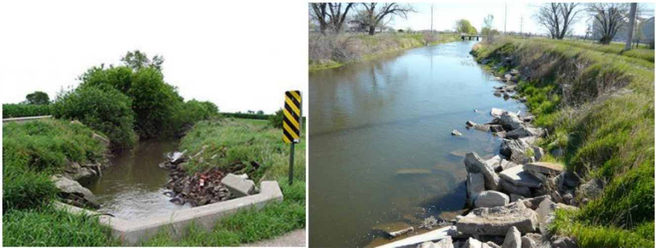
Figure 7 Canals used in the Central Platte MAR, prior (left) and after (right) rehabilitation.
