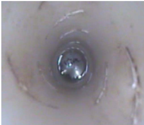
42220053 - Slots (spiral cut) in casing (at 18.6 m - 19.6 m).
