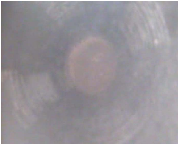
42220027 - Slots in casing (11.5 m - 12.2 m). The clarity of the image is compromised due to the quality of the water in the bore.
