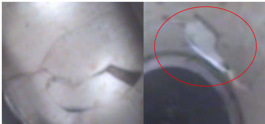
42220019 - Crack in casing at approximately 11.5 m depth.
