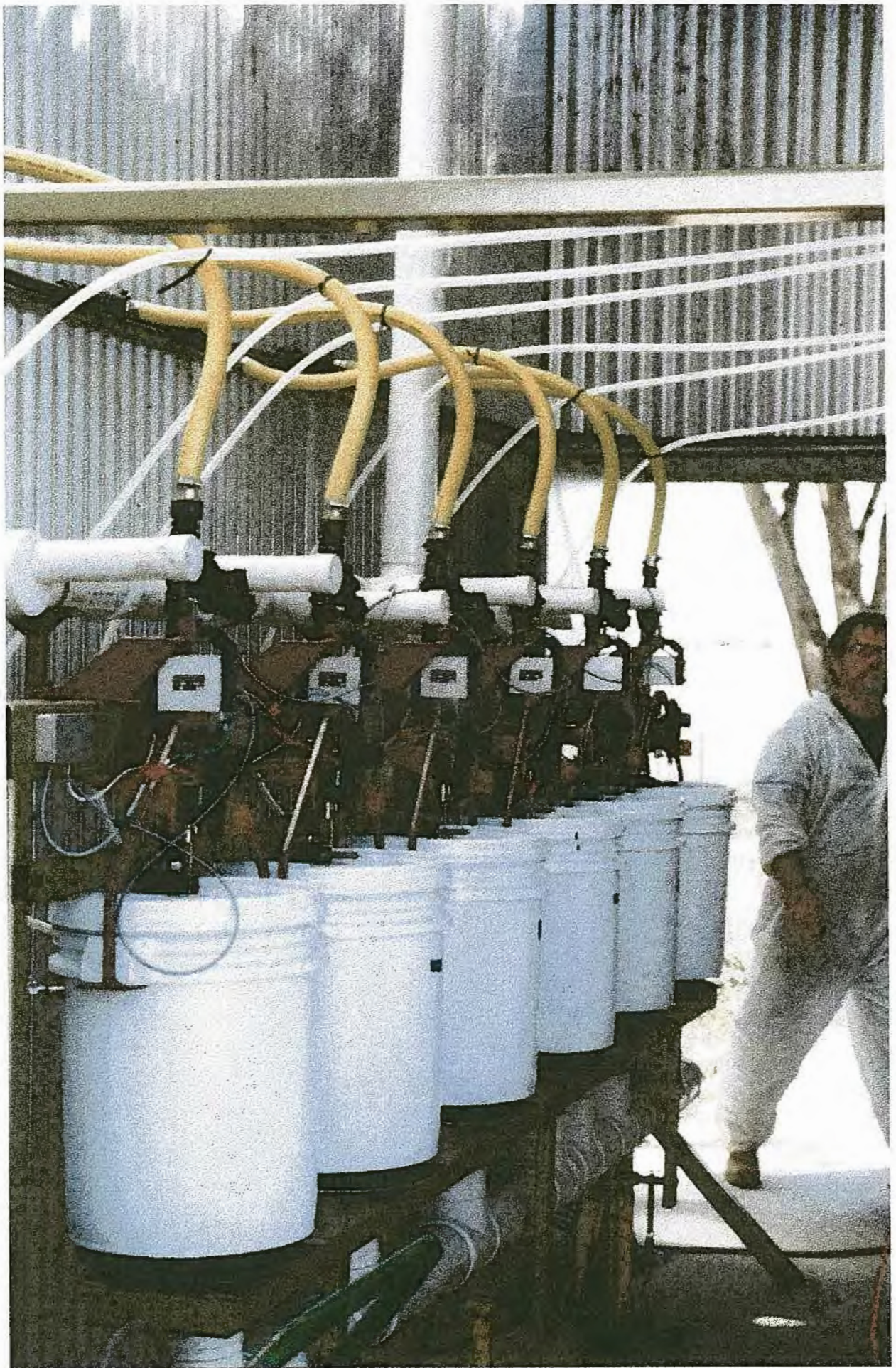
Drum collection system consisting of 12 30-litre drums mounted on load cells.
