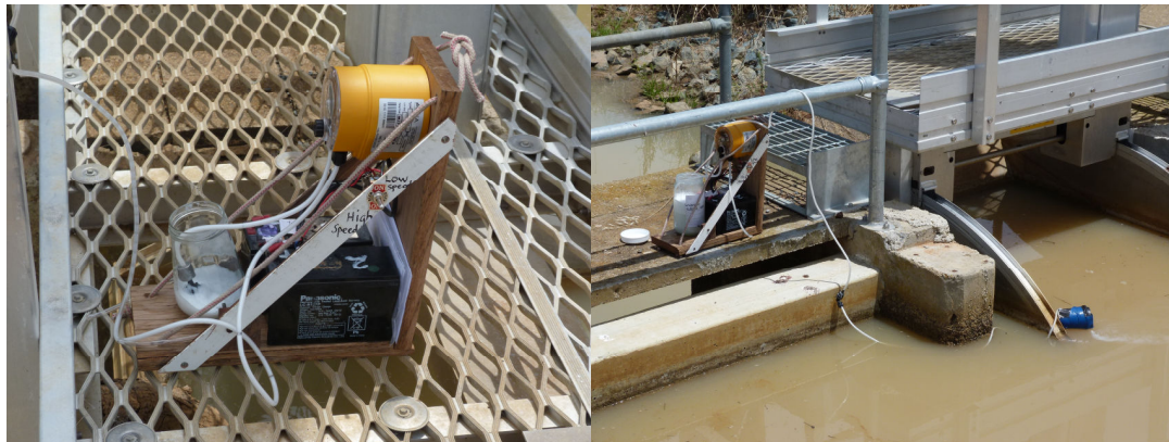
Figure 2.9 – Peristaltic pump installation on an irrigation channel by G-MW
