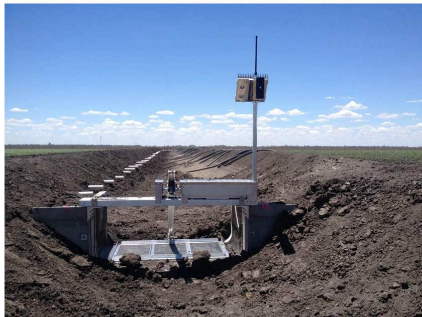
The BayDrive All-in-one in the open position viewed from upstream with the small diameter PTB's through the channel bank on the left
