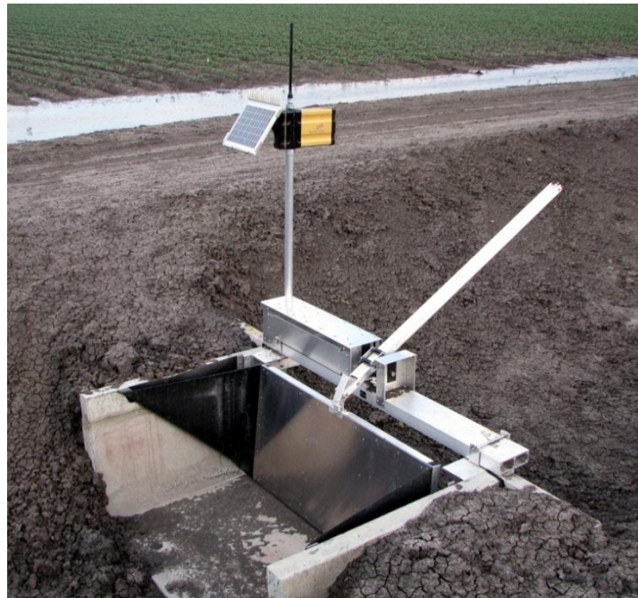
The BayDrive All-in-one in the closed position viewed from downstream
