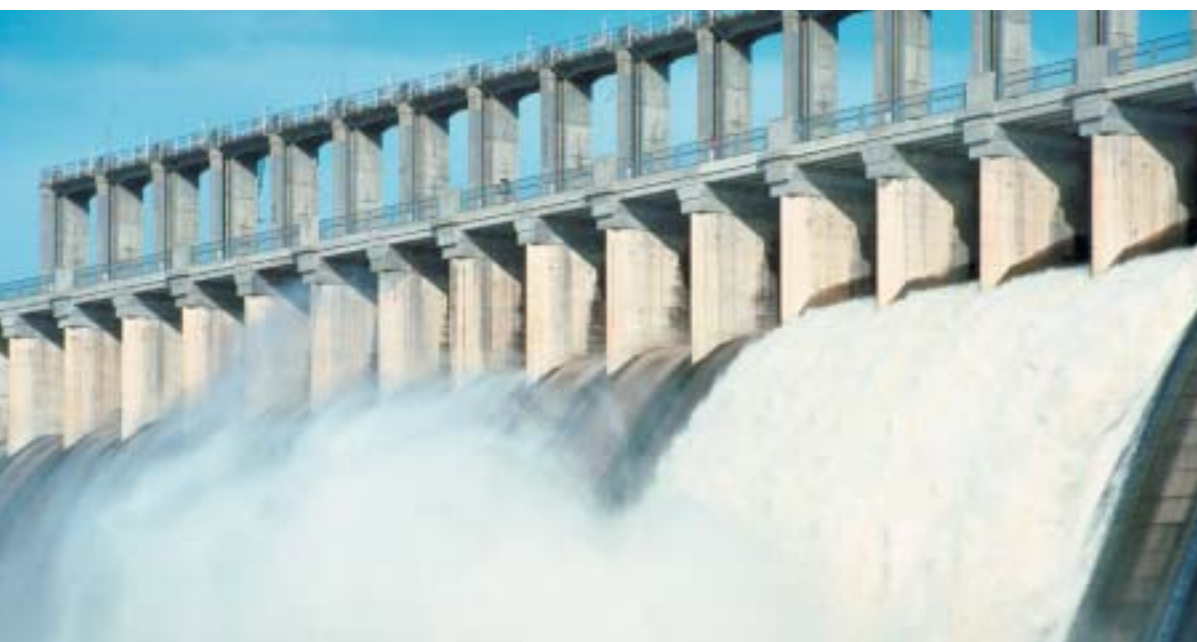
Weirs and dams form barriers to fish migration. Hume Dam. Photo MDBC.
