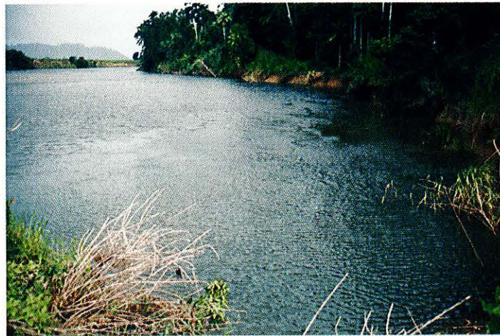
Plate 3 Eroded stream bank prior to construction of pile groynes; showing remnant riparian forest
