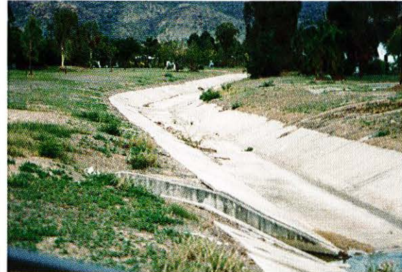
Urban drain in Townsville
