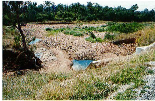
Creek erosion at culvert outlet in Townsville
