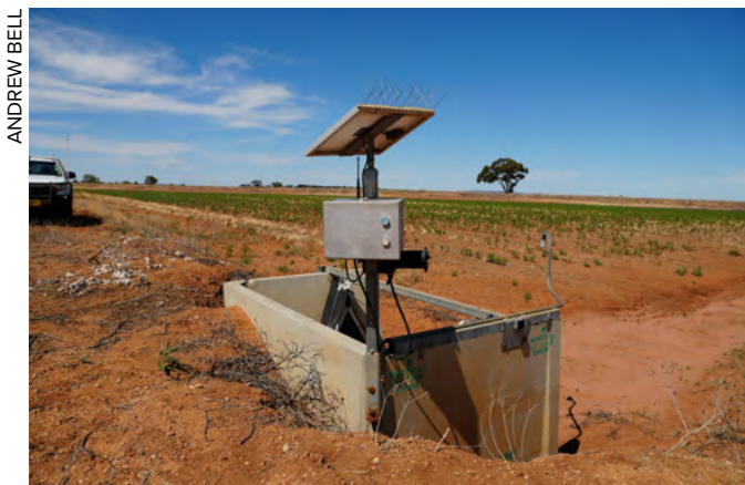
Figure 18: Example of solar powered outlet controller with wired water height sensor and manual override buttons in event of communication failure.
