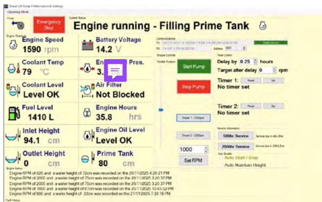
Figure 20: Top: Example of remote pump controller with manual override buttons. Bottom: Example of user interface for monitoring pumper operations.
