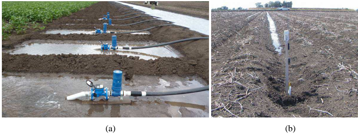
Figure 6.3: (a) Inflow meters installed in-line with siphons; and (b) advance meter
