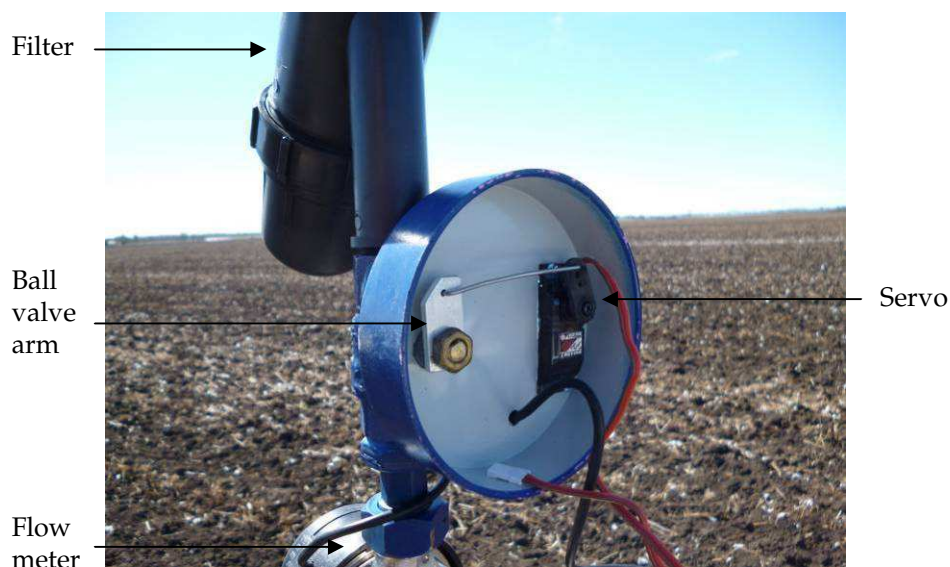
Figure 6.2: Hardware used for adjusting flow rate during irrigation events
