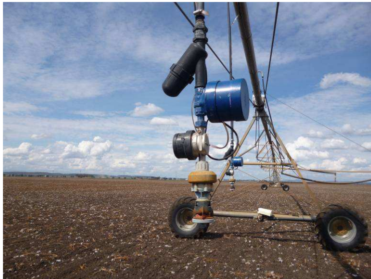
Figure 6.5: Water filter, flow meter and controllable ball valve on outlet of centre pivot irrigation machine
