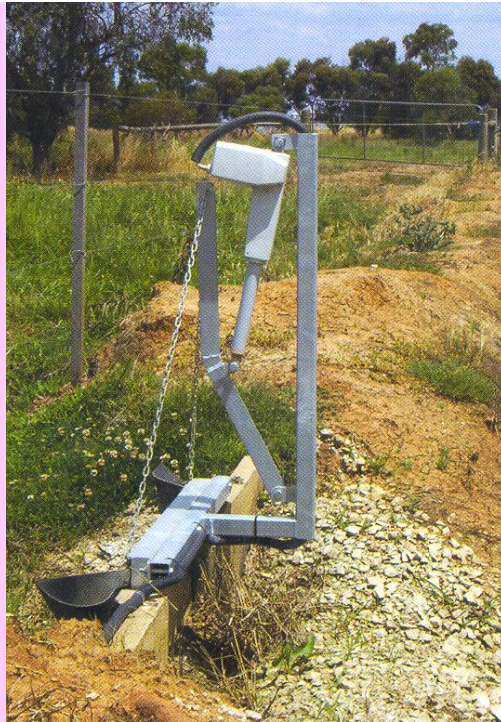
Actuator on bay inlet structure
