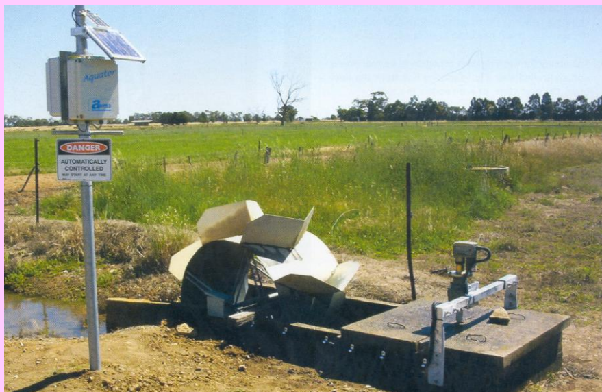
Automated Dethridge meter wheel
